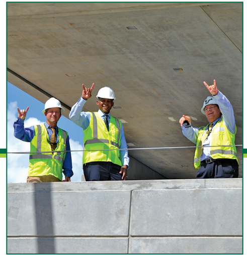
On the Job: Brian Laverty, Facilities Project Manager; VP Williams; and Steve Lafferty, Assistant Director - Design & Construction checking the progress at the P3 construction site.
