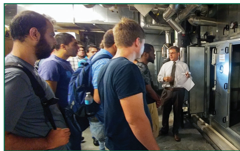
Toufic Moumne shows USF engineering students air-handlers in the Rec Center mechanical room.
